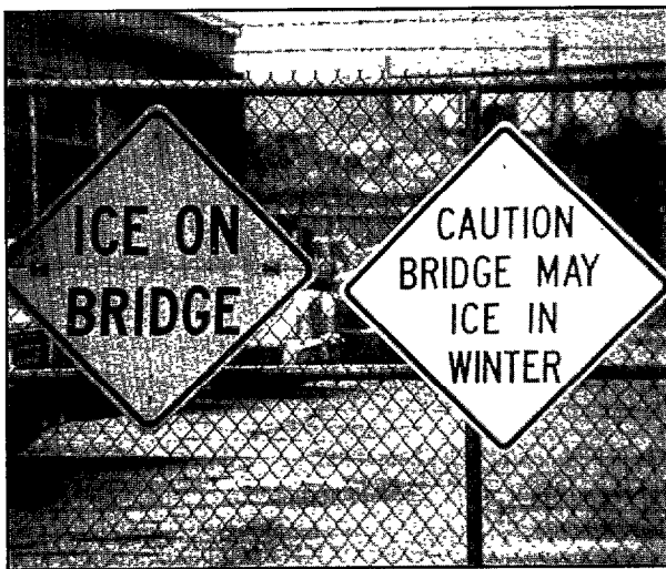
Figure 85. Warning sign with deteriorated retroreflectivity
